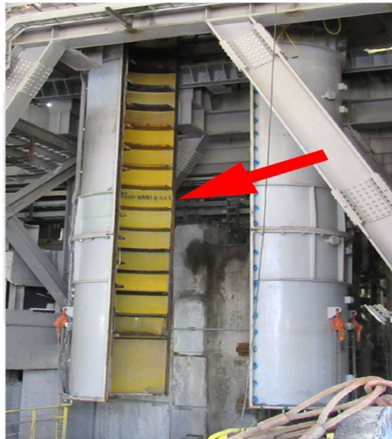
Figure 14—HIGmill liner wear indicated in the mill chamber
