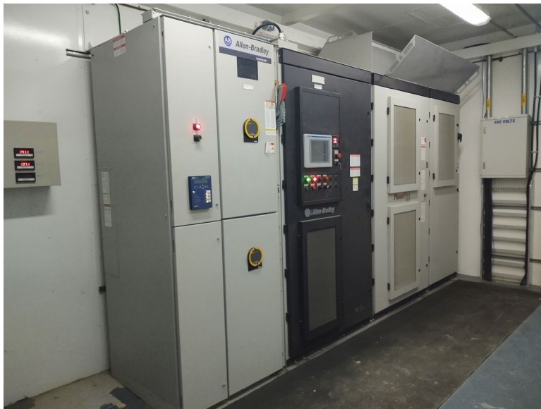
Figure 8 – Ball mill VSD
