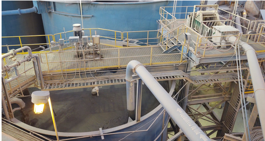
Figure 9 – Trash screen and rougher tank
