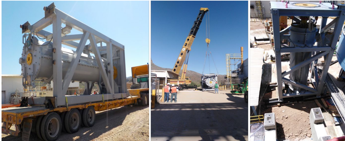
Figure 19 – HIGmill installation and commissioning
